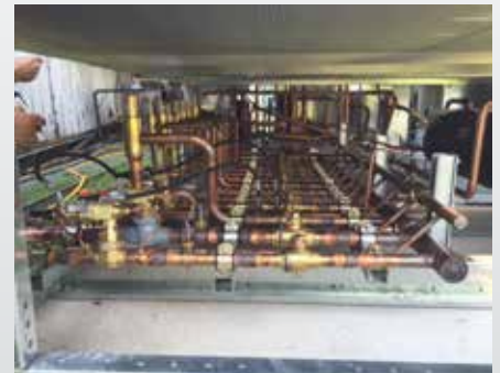
Refrigeration Circuits (below a condenser of a LINK+)
