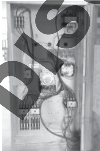
Large Electrical Panel
