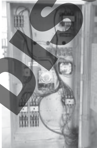
Large Electrical Panel
