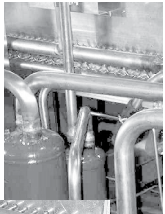
Pre-formed internal piping
